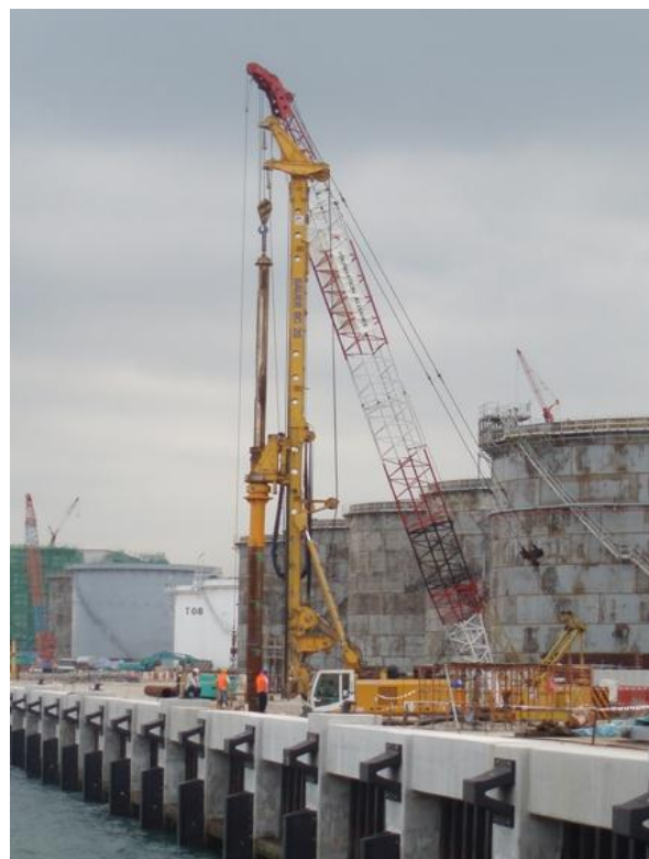
Installation of steel tubular pipe piles upto 36.6m by Bauer BG28 rotary drive adaptor & preboring (vibration free) next to new quay wall & farm tanks
