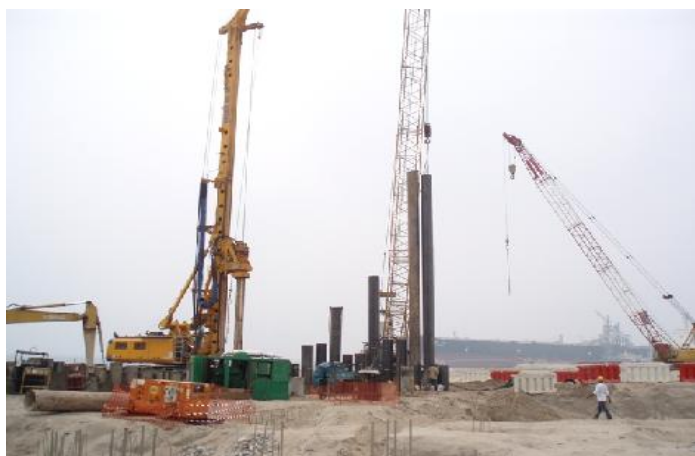
Installation of steel tubular pipe piles upto 36m by preboring & vibro hammer for Admin Building's protection
